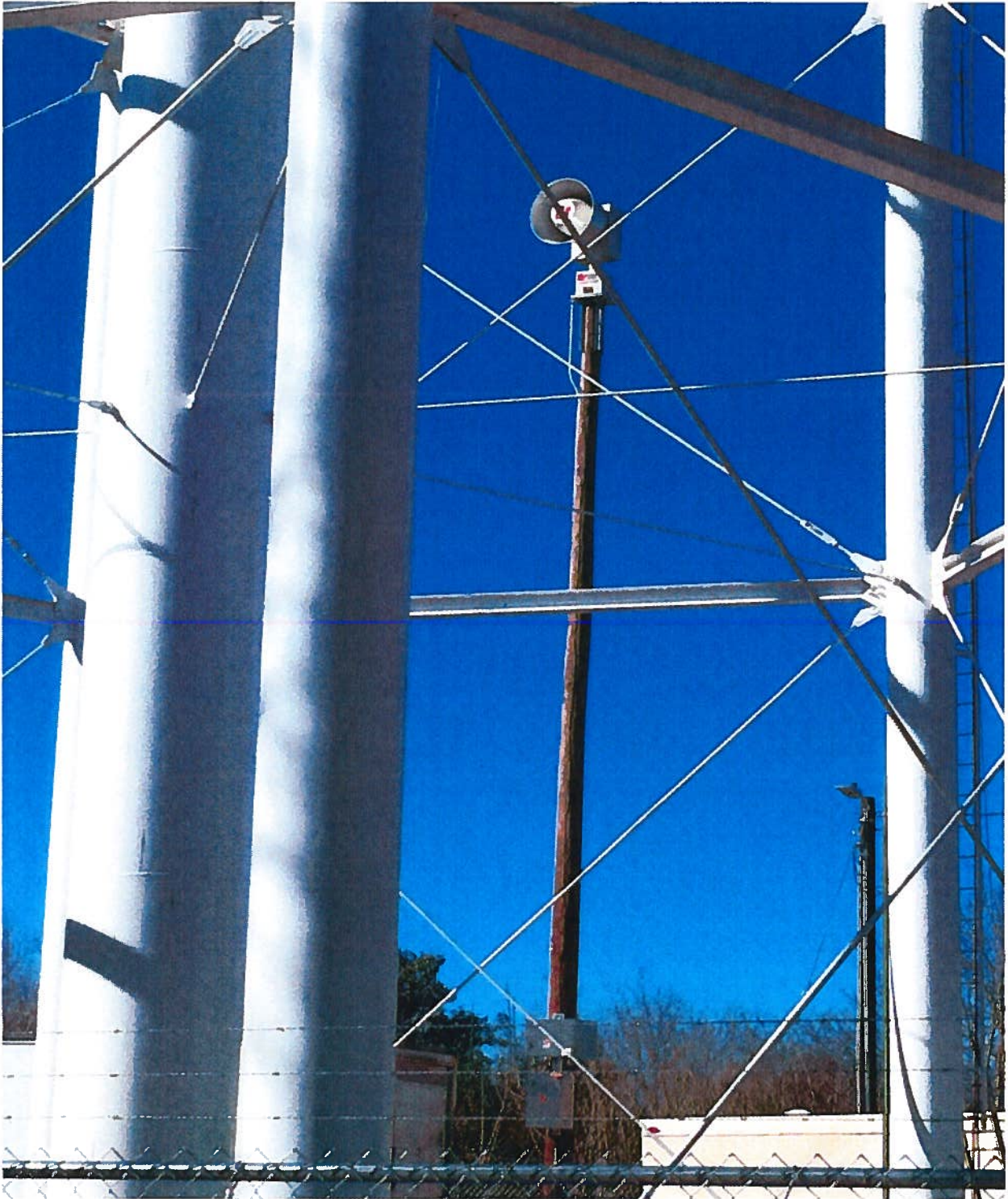
Figure "C-3" – MARTINDALE SIREN SITE 2
