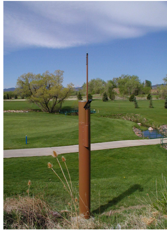
Packaged Pressure Transducer Station, City of Loveland, CO
