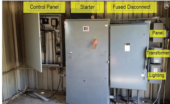
Existing Electrical Equipment & Control Panel
