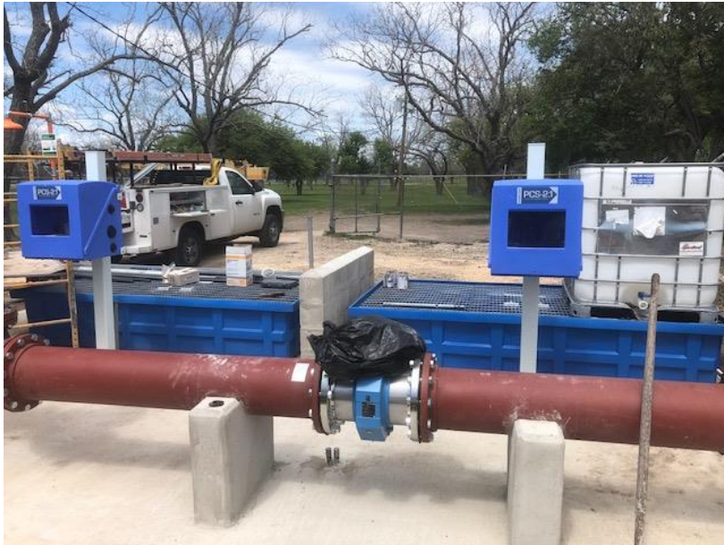
NaOCl and LAS Storage Tanks and Feed Pumps
