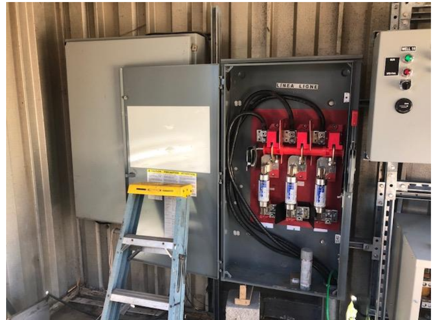
Motor Control Center
