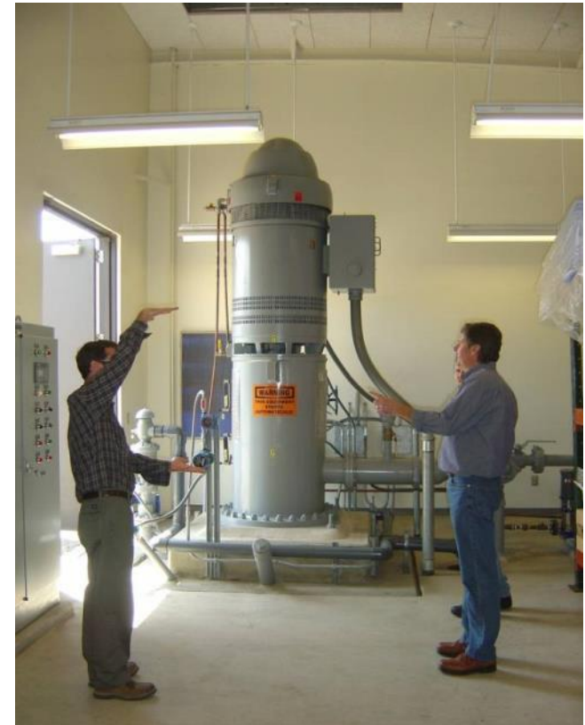
Calleguas MWD, California
