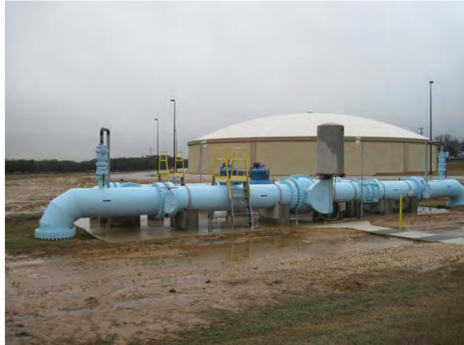
SAWS Flow Control Facilities and Ground Storage Reservoir at Twin Oaks WTP and ASR Wellfield
