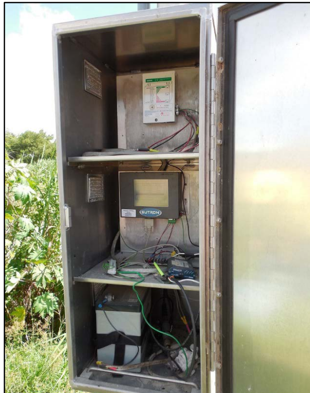
Figure 10. CAMS 793. View of control box. Battery on bottom shelf and control/communication system on middle shelf. Photo by SDI Engineering, LLC. September 29, 2014.
