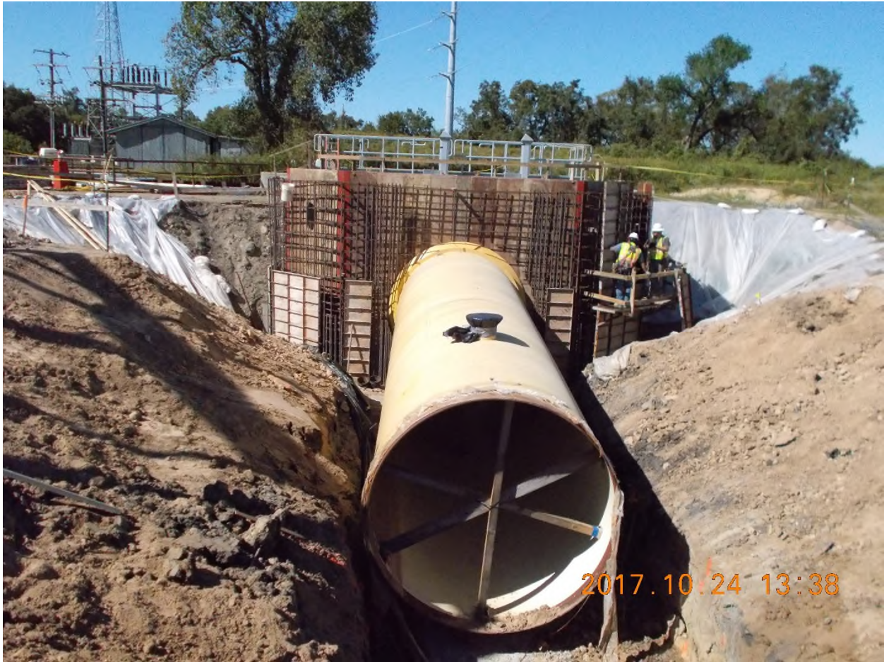
Figure 4-23. Construction of Canal Inlet Structure and First Segment of River Return Pipe
