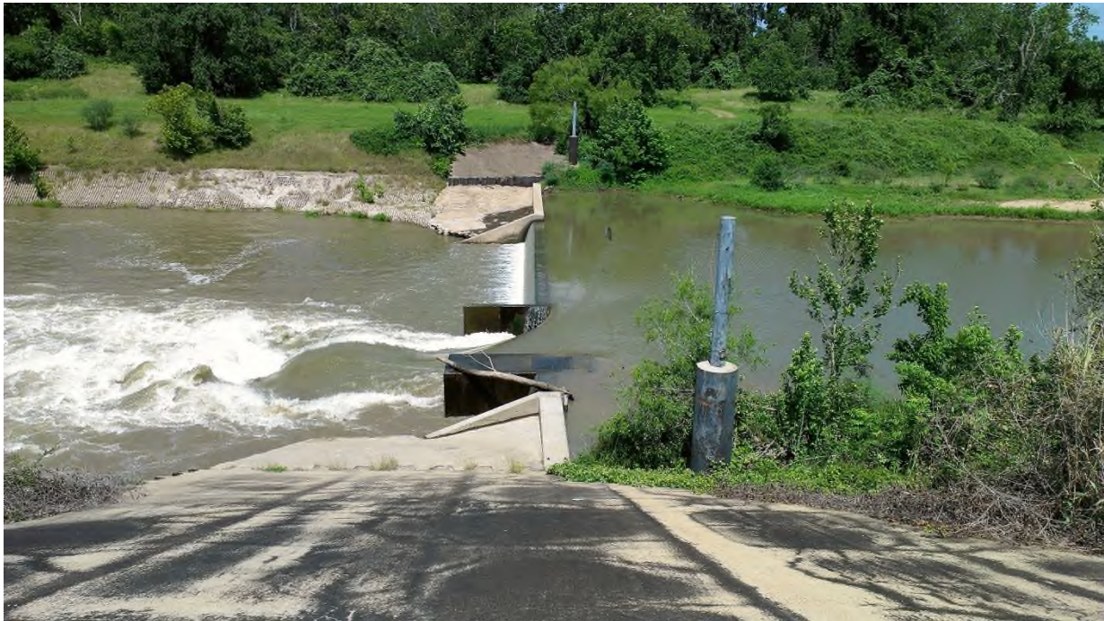
Figure 3-23. Lane City Dam, Standing on Top of Left (East) River Bank Looking West
