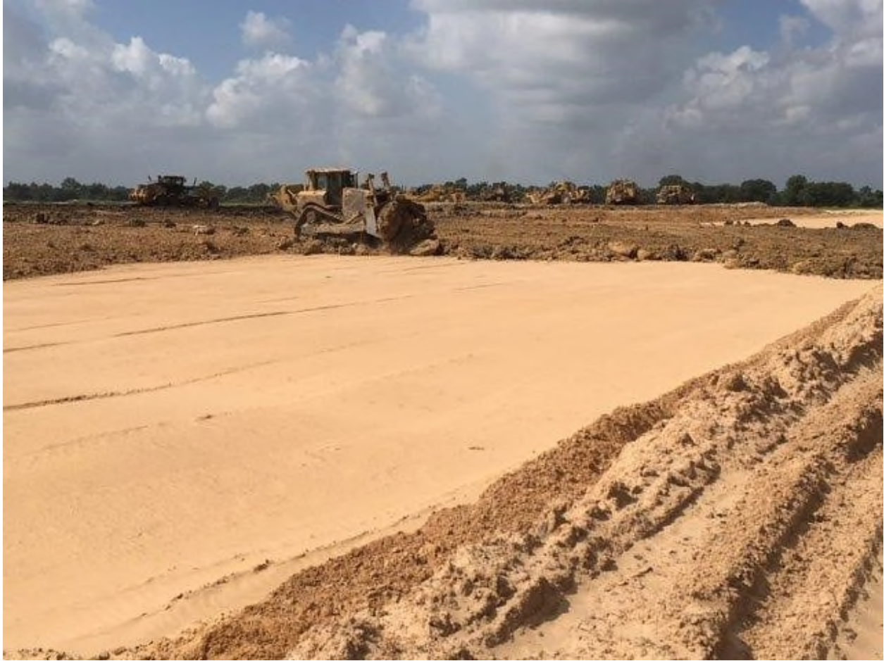
Figure 3-16. Blanket Drain Complete and Initial Soil Lifts Over Blanket Being Placed on South Embankment
