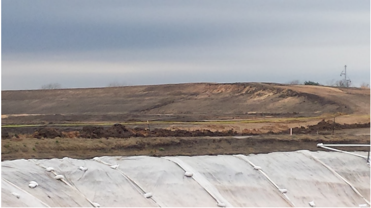
Figure 3-13. Looking West from the Inlet/Outlet Excavation at the Northwest Corner of the Embankment at Full Height
