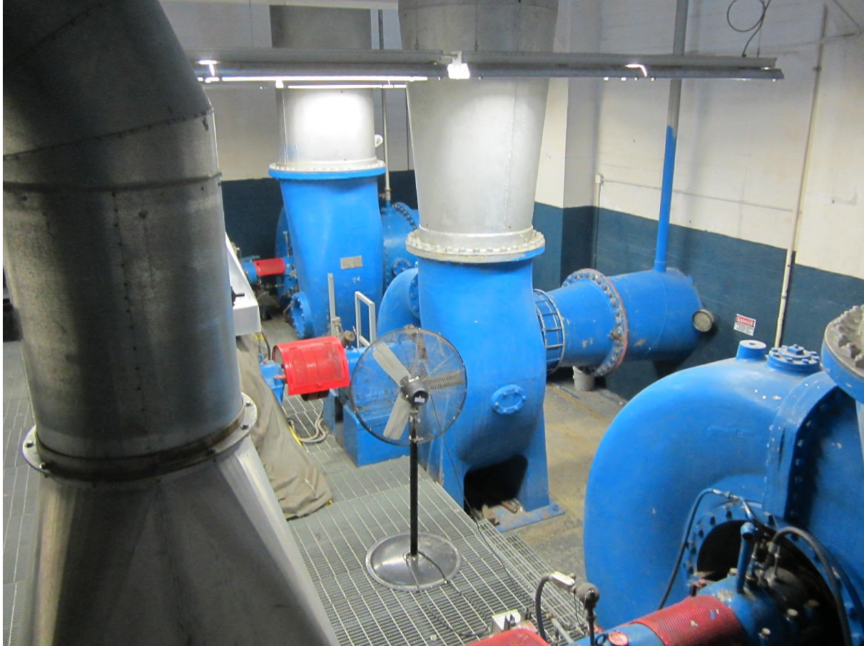
Figure 3-3. Pumps Inside HPS Building
