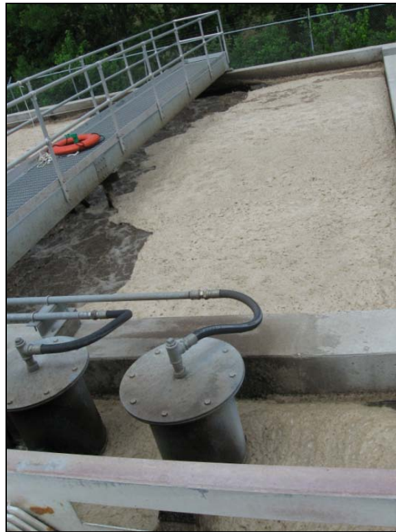
Figure 1.20 Pre-mix Basin and Aeration Basin at the Anna WWTP
