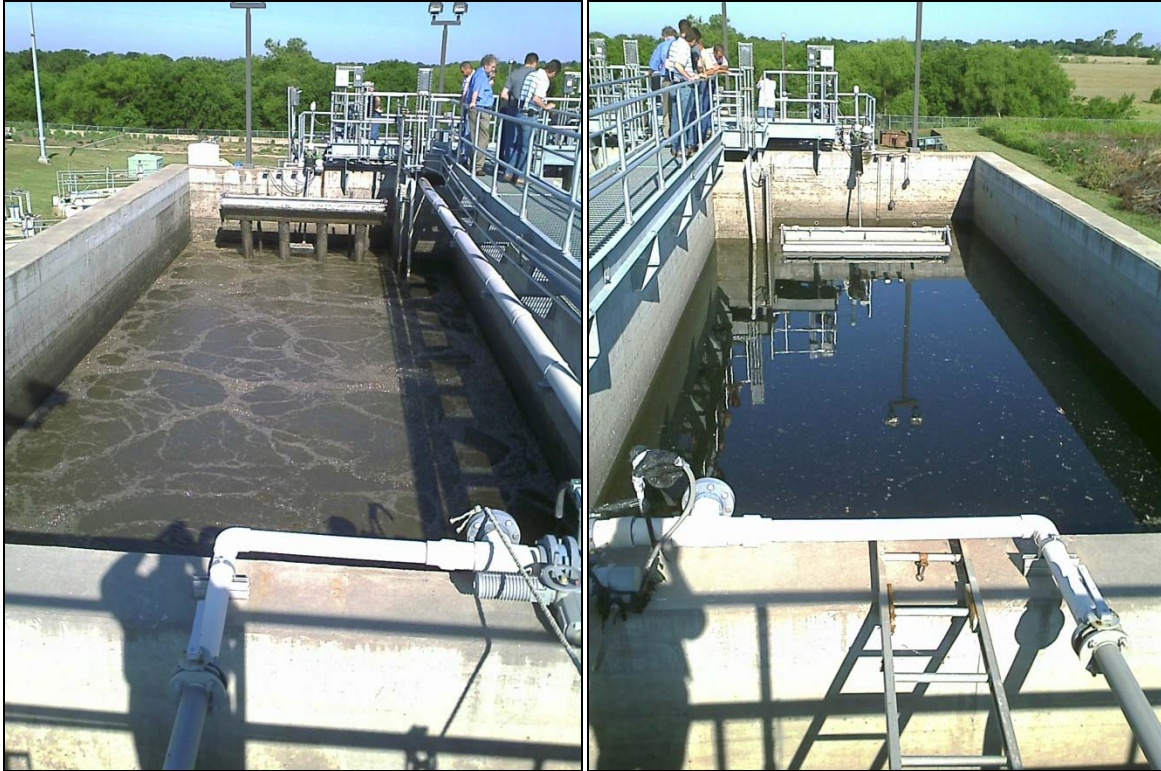
Figure 1.5 Parallel Basins in the ICEAS at the Celina WWTP
