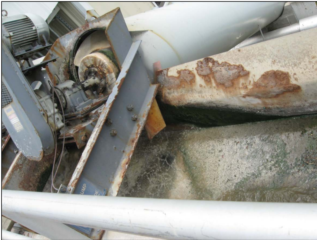
Figure 1.25 Visible Corrosion on the Influent Screw Pumps at the Anna WWTP
