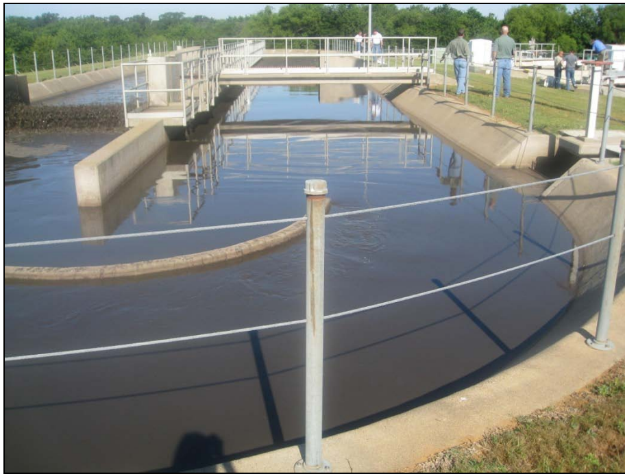
Figure 1.4 Oxidation Ditch at the Celina WWTP
