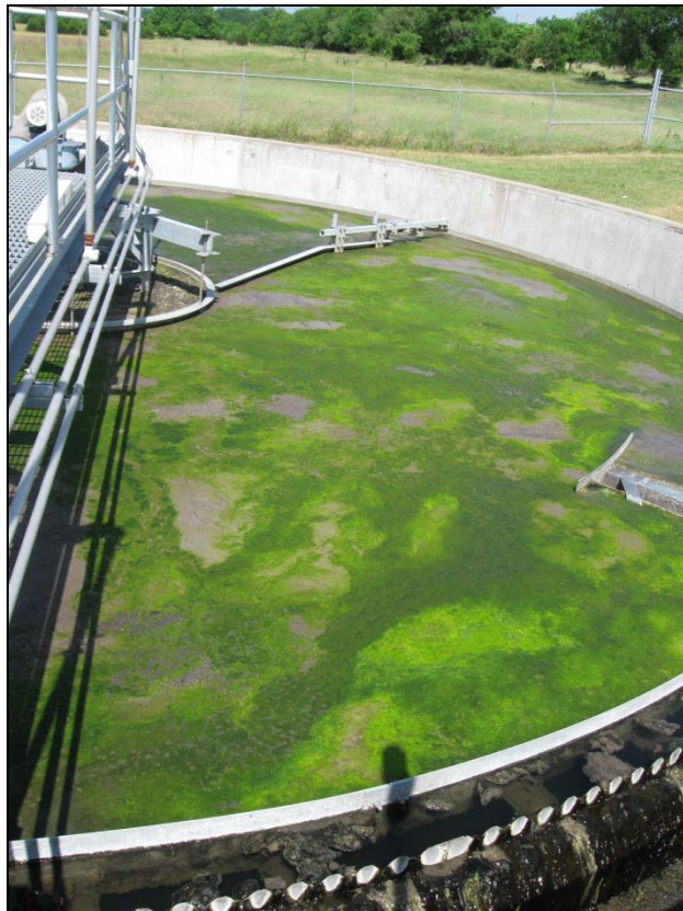
Figure 1.15 Secondary Clarifier with Non-Operational Skimmer
