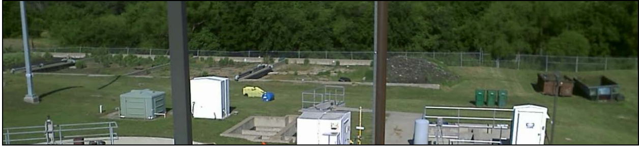
Figure 1.6 Solids Dewatering Beds at the Celina WWTP
