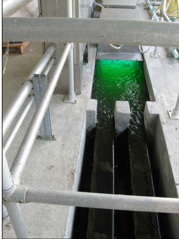
Figure 1.12 UV Disinfection Channel at the Van Alstyne WWTP
