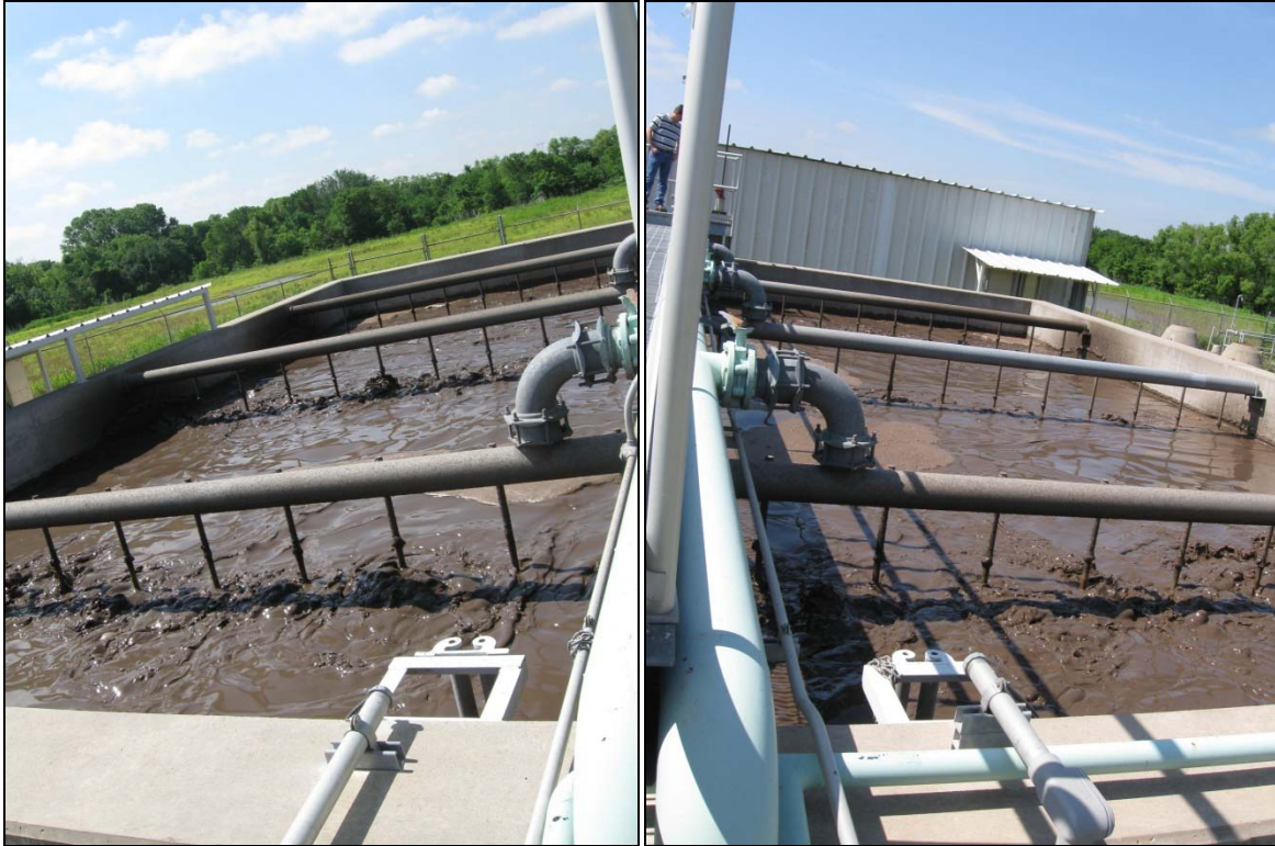
Figure 1.13 Aerobic Solids Holding Tank At The Van Alstyne WWTW
