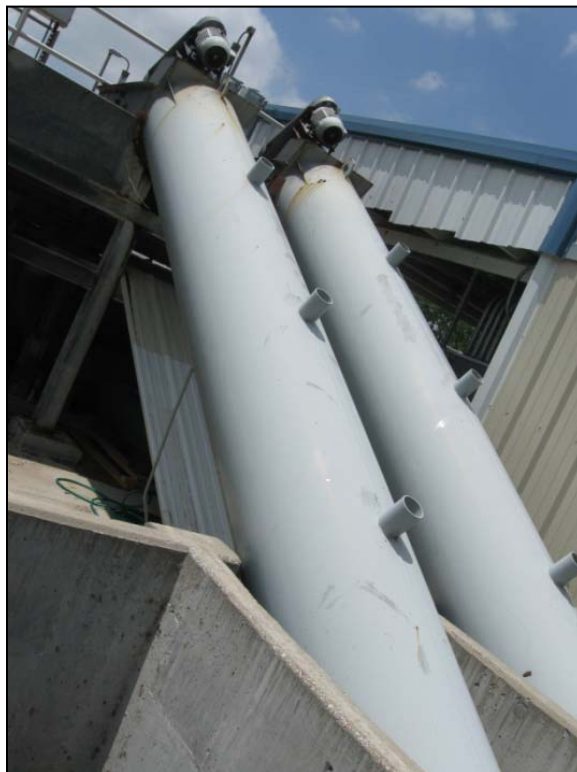
Figure 1.19 Influent Screw Pumps at the Anna WWTP
