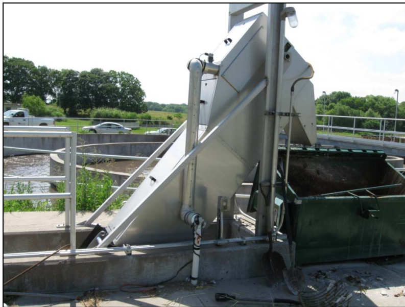
Figure 1.10 Influent Fine Screen at the Van Alstyne WWTP
