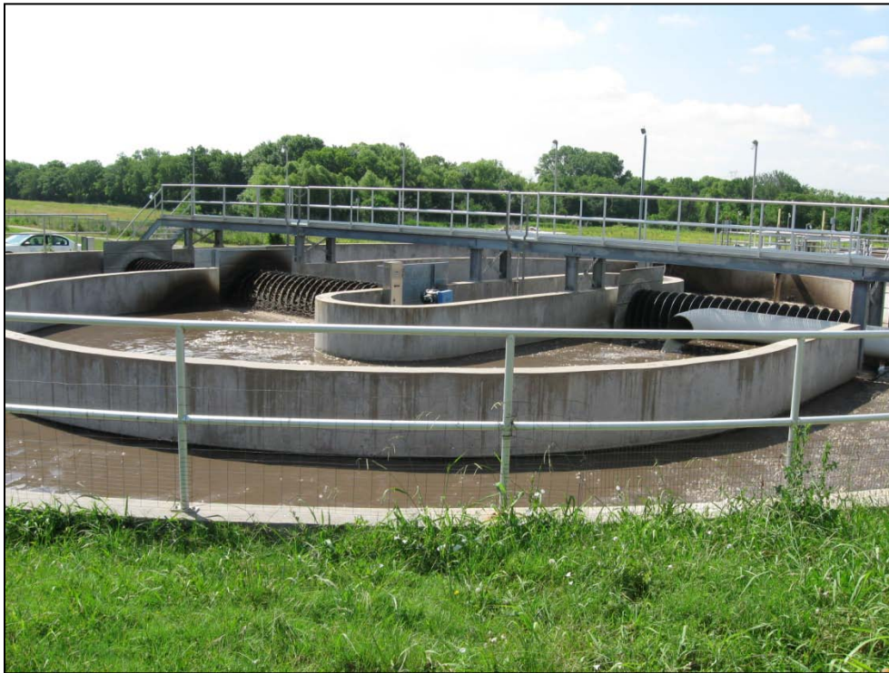
Figure 1.11 Orbal ® Oxidation Ditch at the Van Alstyne WWTP
