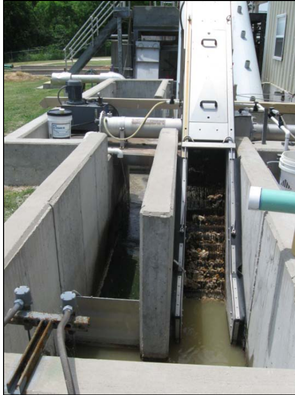
Figure 1.18 Influent Fine Screens at the Anna WWTP
