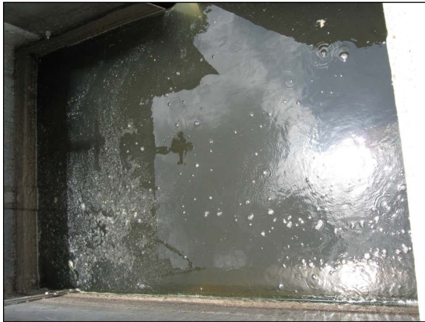
Figure 1.23 Surface Grease Present in the Final Effluent Flow Box
