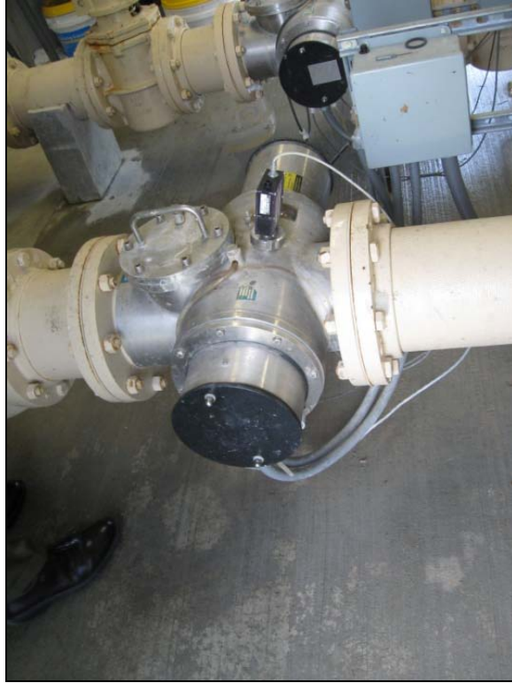
Figure 1.22 In-pipe UV System at the Anna WWTP
