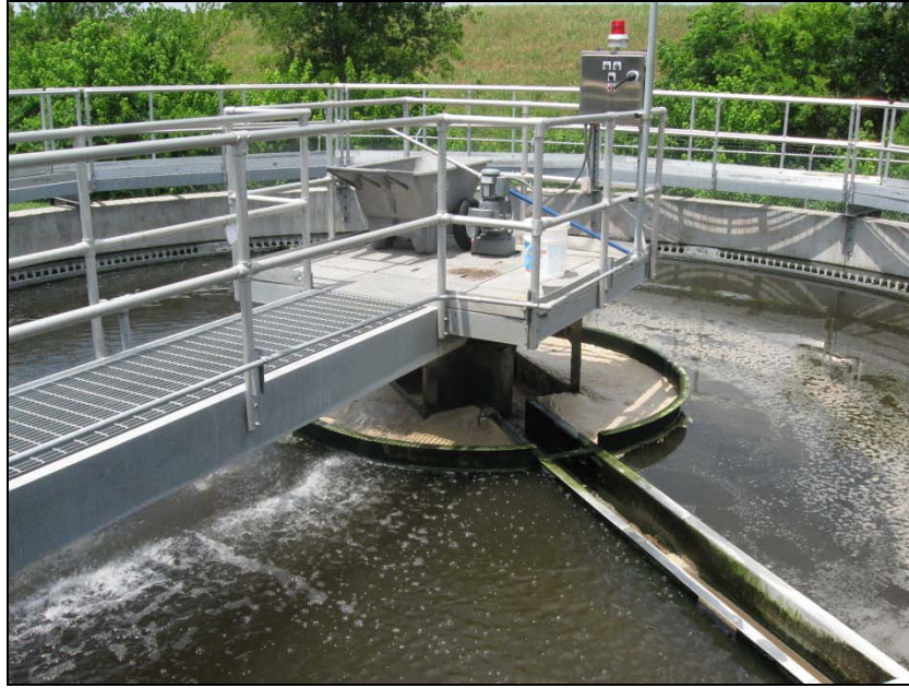
Figure 1.21 Secondary Clarifier at the Anna WWTP
