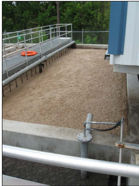
Figure 1.24 Thickener and Aerobic Holding Tank at the Anna WWTP
