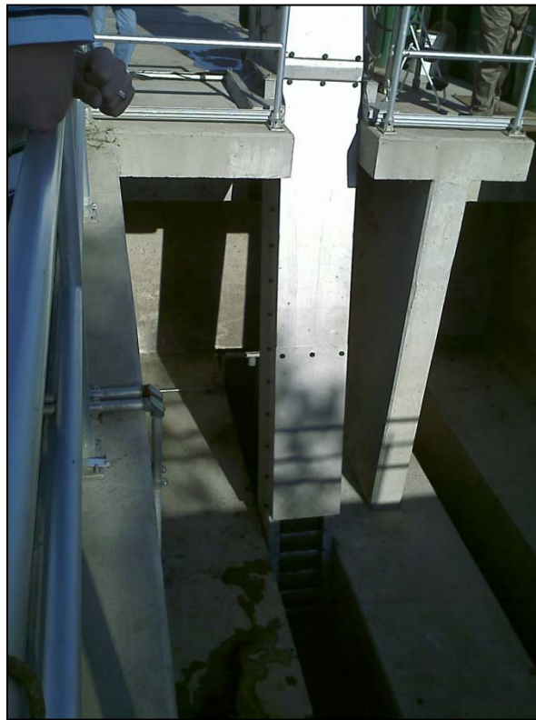
Figure 1.3 Influent Fine Screens at the Celina WWTP
