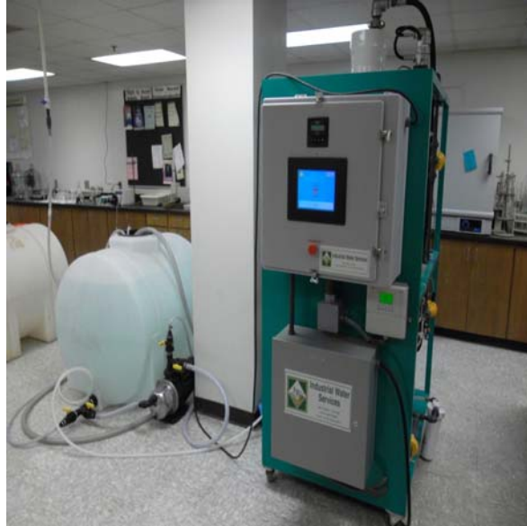
Figure 2-2. Pilot RO system control panel and batch feed tank.
