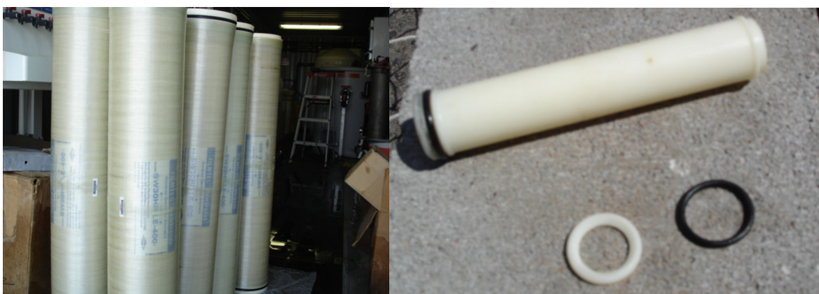
Figure II-16: RO membranes (left), broken interconnector for RO spacer membrane (right).
