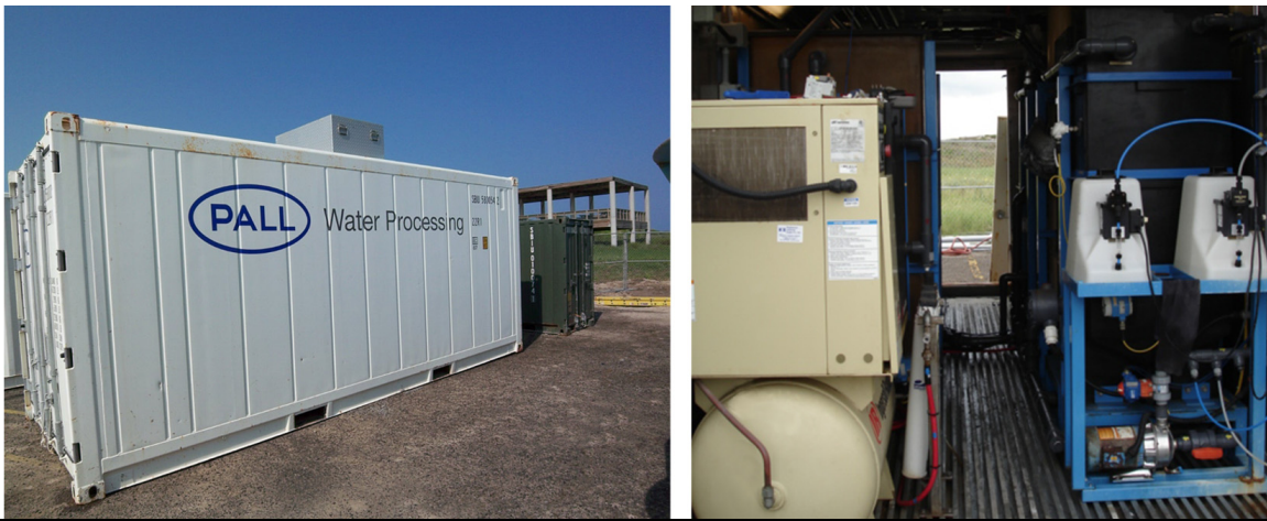
Figure II-11: Pall pretreatment container (left), interior of Pall pretreatment container (right).
