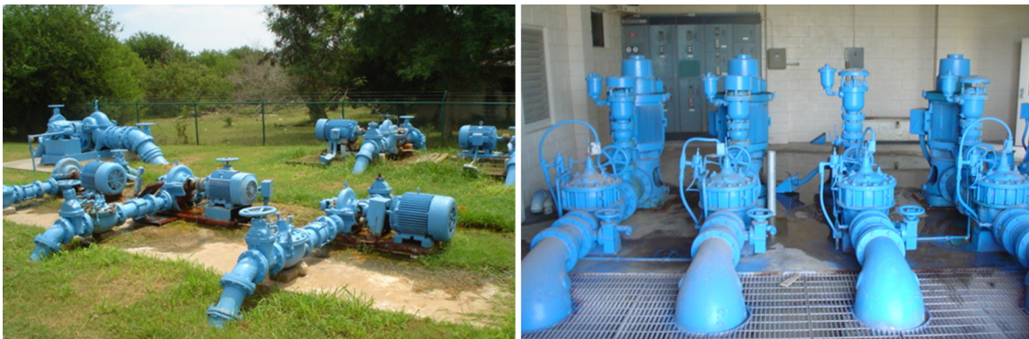
Figure I-9: WTP #1 (left) and WTP #2 (right).
