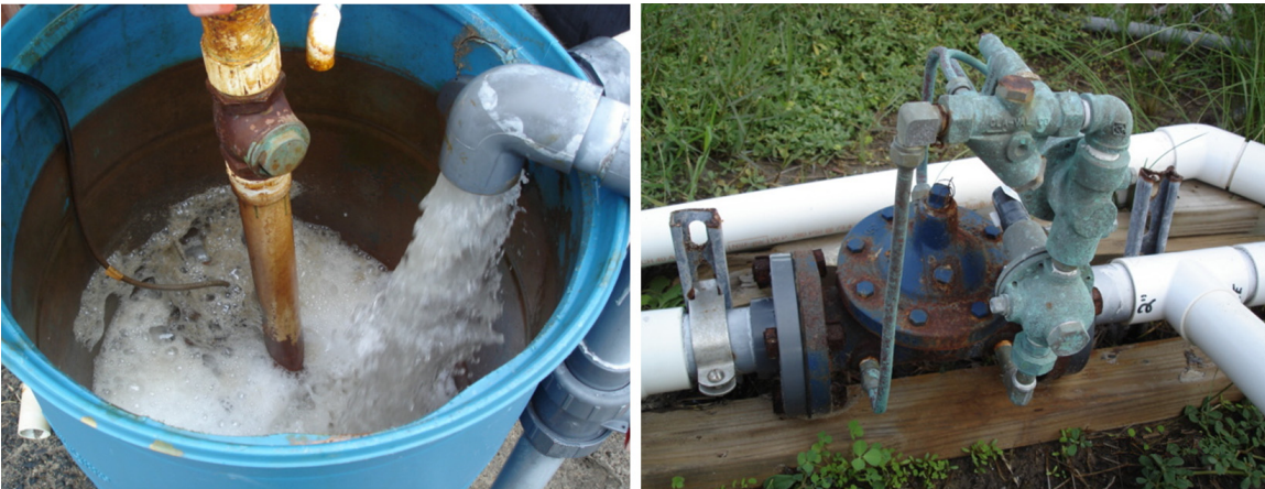
Figure II-8: Raw water coming in from Gulf of Mexico (left), pressure relief valve (right).
