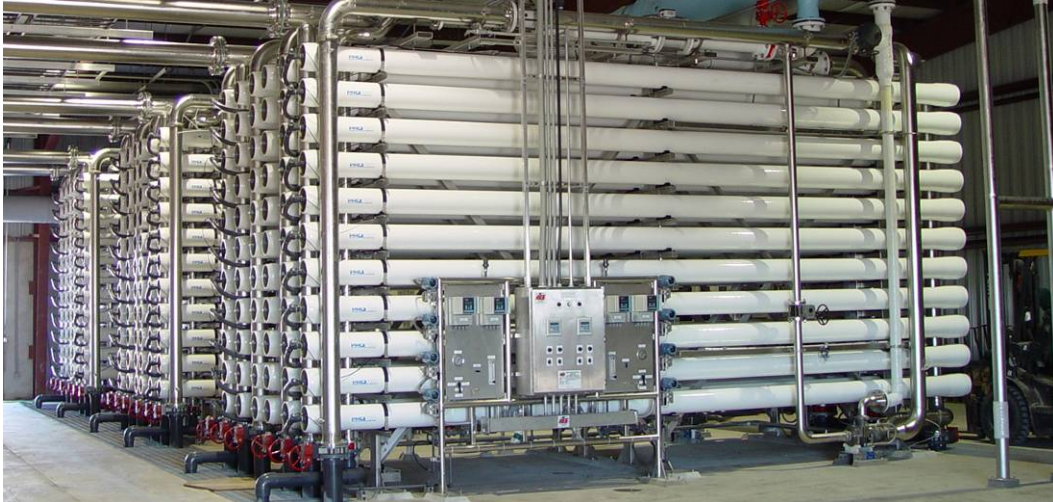
Figure I-42: SRWA brackish desalination plant RO units.
