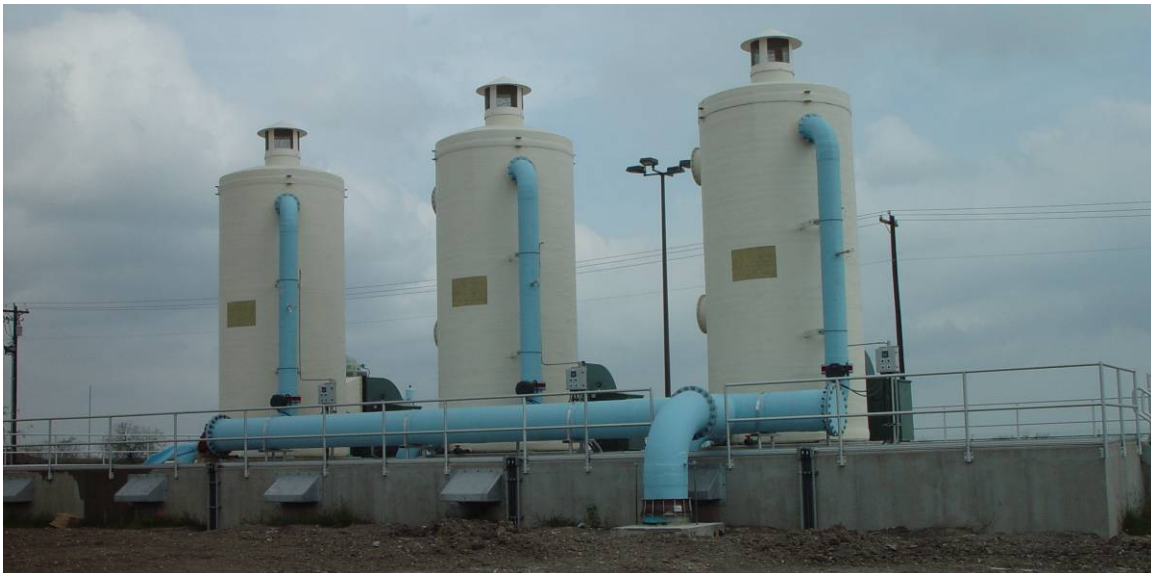
Figure I-43: SRWA brackish desalination plant transfer pump station and degasifier units.
