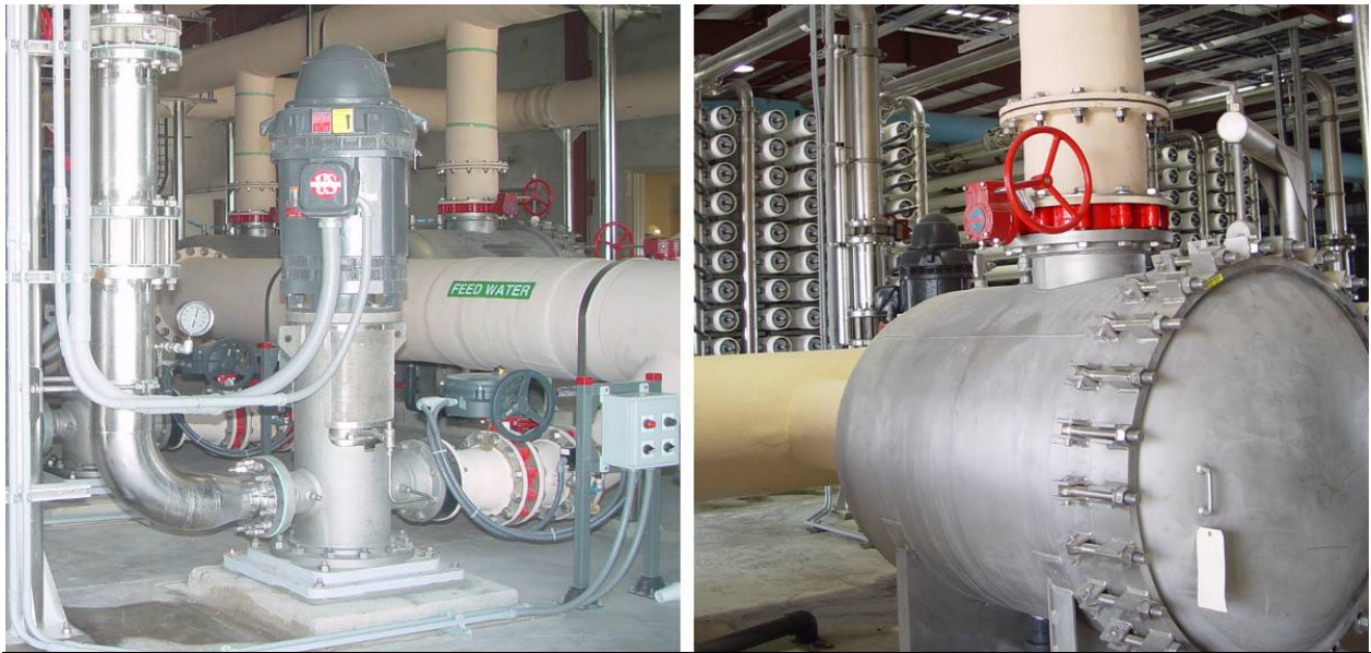
Figure I-40: Southmost Regional Water Authority brackish desalination plant high pressure RO feed pump (left) and cartridge filter (right).
