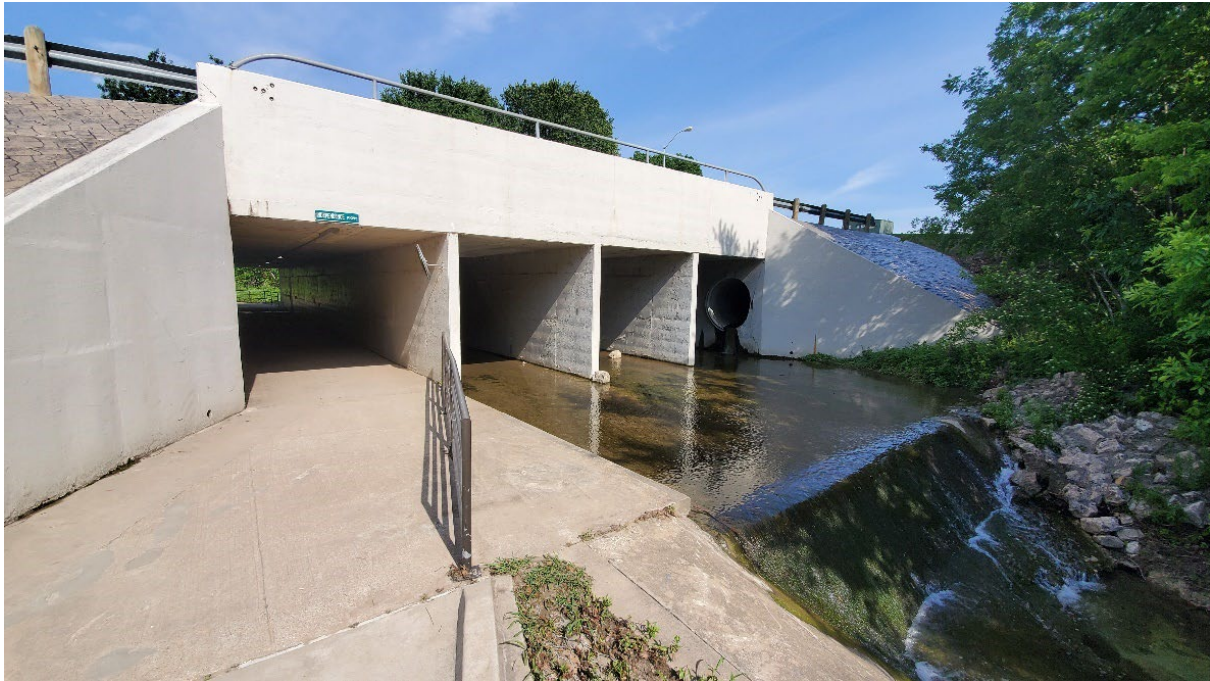
Figure 2.52: Staged or Tiered Culvert Design Used in North Texas with Multiple Culvert Sizes and Flow Elevations
