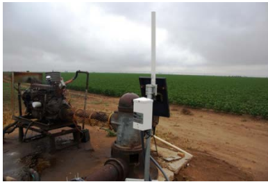
Surface turbine irrigation well
