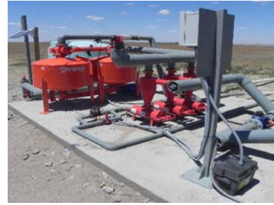
SDI filtration system
