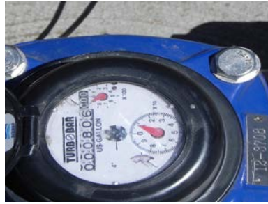
Water meter on system
