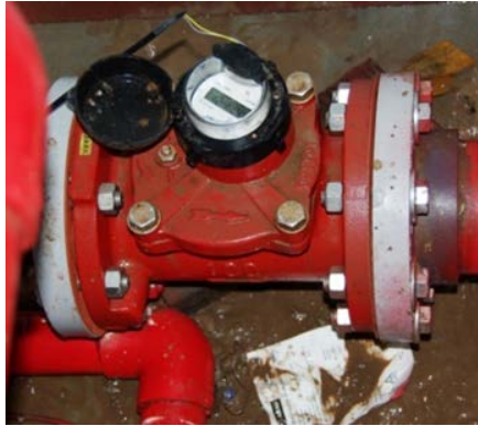
Meter on SDI drip system
