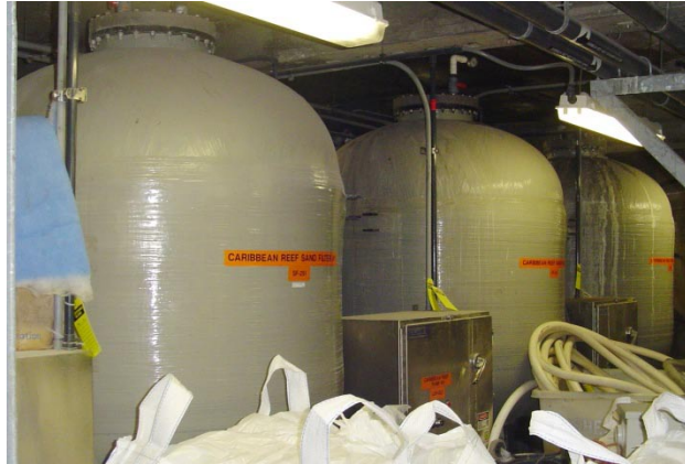
Figure 12. Large Aquarium Sand Filters
