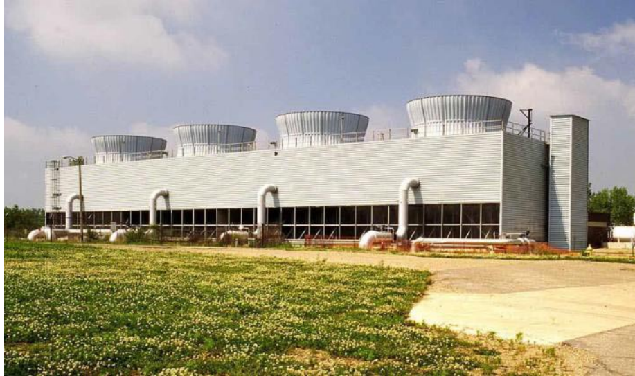
Figure 3. Marley Counter-flow Towers
