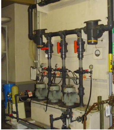
1 2 Figure 7. Fume Scrubber for a Microelectronics Lab
