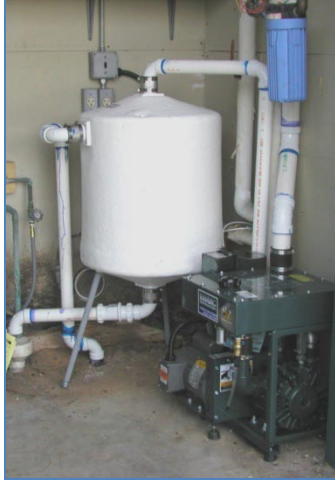
1 2 Figure 5. A Dry Vacuum System at a Dental Office 3 4
