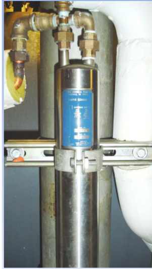
1 2 Figure 10. Boiler Water Sampler Device 3
