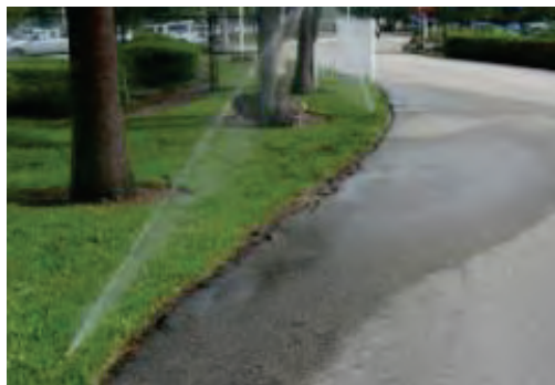
Figure 49. Sprinklers with a poor wetting pattern.
