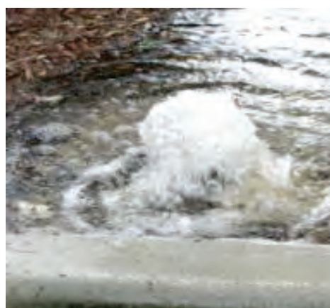
Figure 50. Broken sprinkler head creating a “geyser.”
