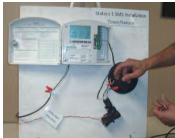
Figure 58. A demonstration of proper wiring of a soil moisture sensor.
