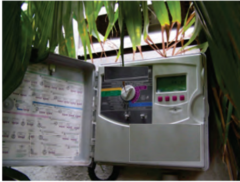
Figure 59. A smart irrigation system control box.
